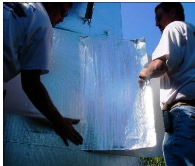
Pull release film from behind membrane and continue to press into place.
